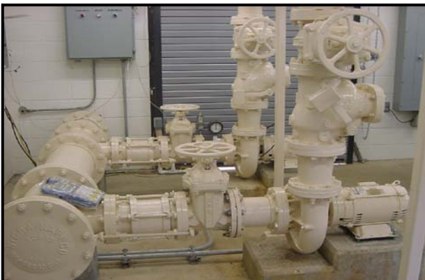
RAW WATER PUMPS
