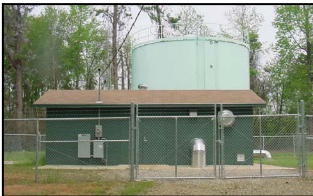
PUMP STATION & 100,000 GALLON GROUND TANK
