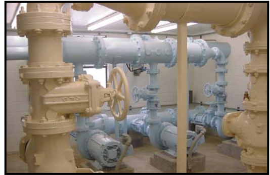
HIGH SERVICE PUMPS
