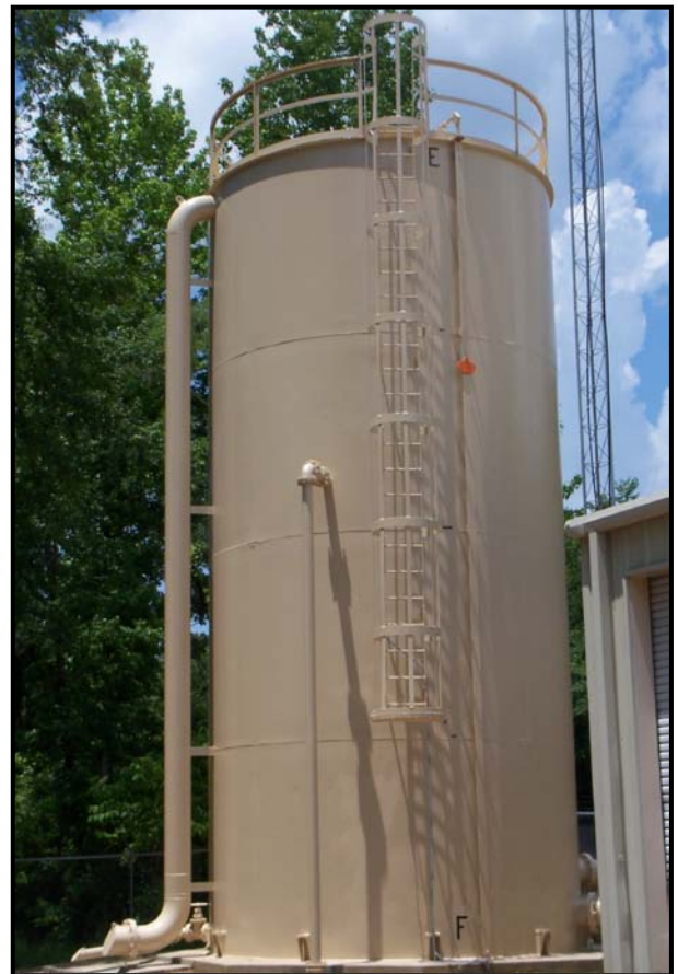
50,000 GALLON RAW WATER STORAGE TANK
