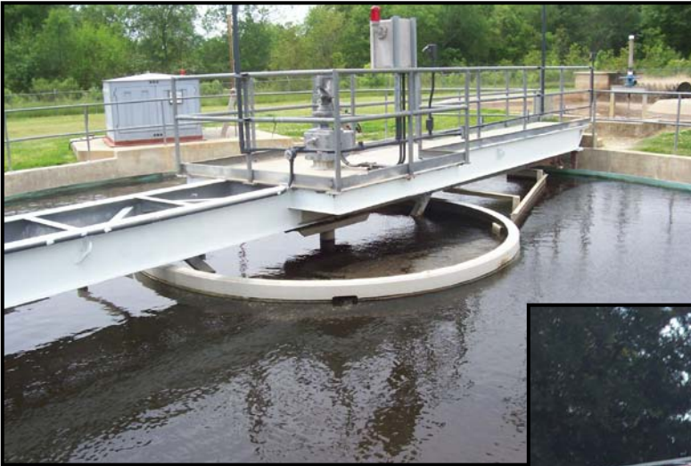
ACTIVATED SLUDGE TREATMENT
